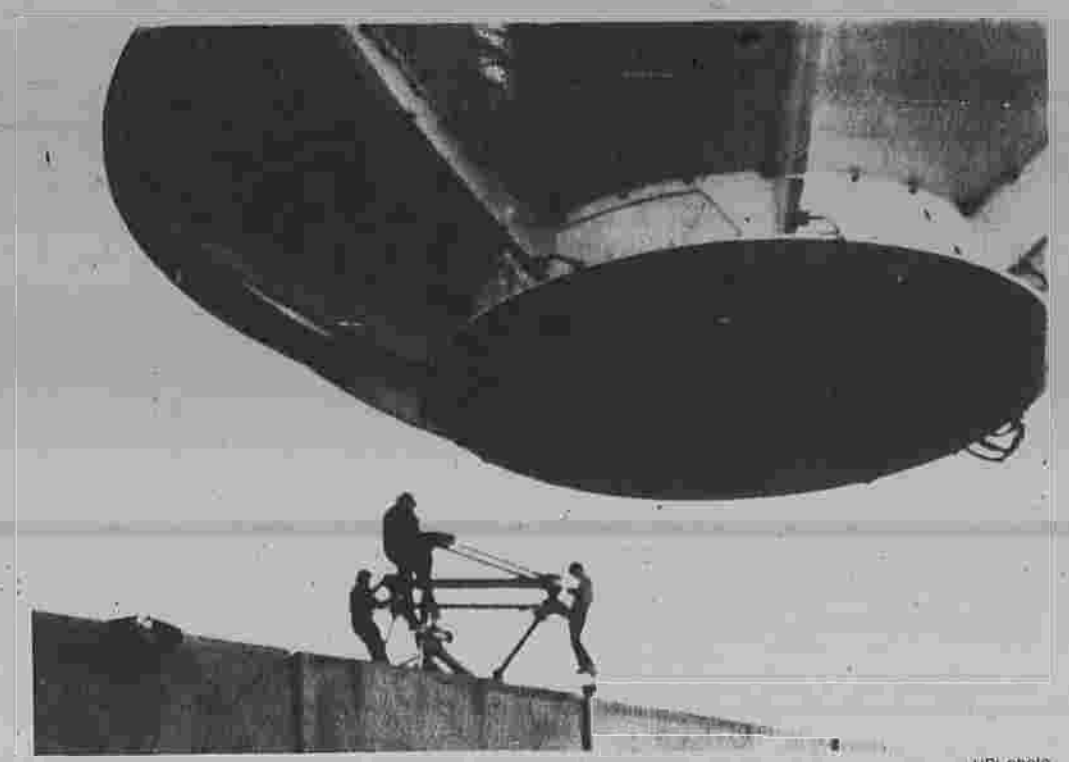
No, it's not a 'close encounter' It's not a visit from outer space by a flying saucer. It's just the installation of an 18-foot, 4.5-ton dish antenna on the roof of the Travelers Insurance Co. Data Center in Hartford Wednesday for contact, via satellite, with the firm's alternate data processing facility under construction near Atlanta, Ga.
